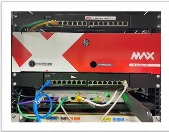
Fig 3. CMS Site Controller
